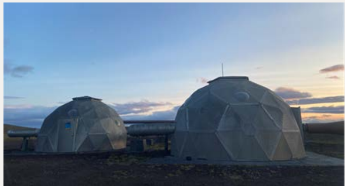
Ice houses (iglos) covering the producing wells in Krafla
